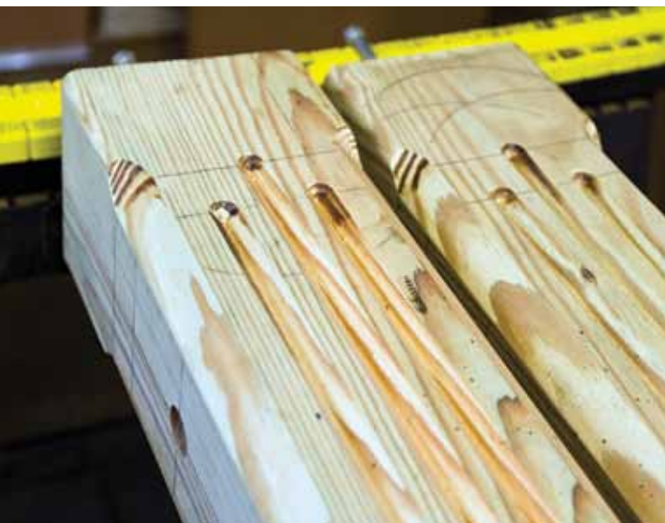
With the fluting, chamfering and rounding-over complete, the last milling step requires drilling holes in the posts to accept the brackets we use to support the sign panels.
