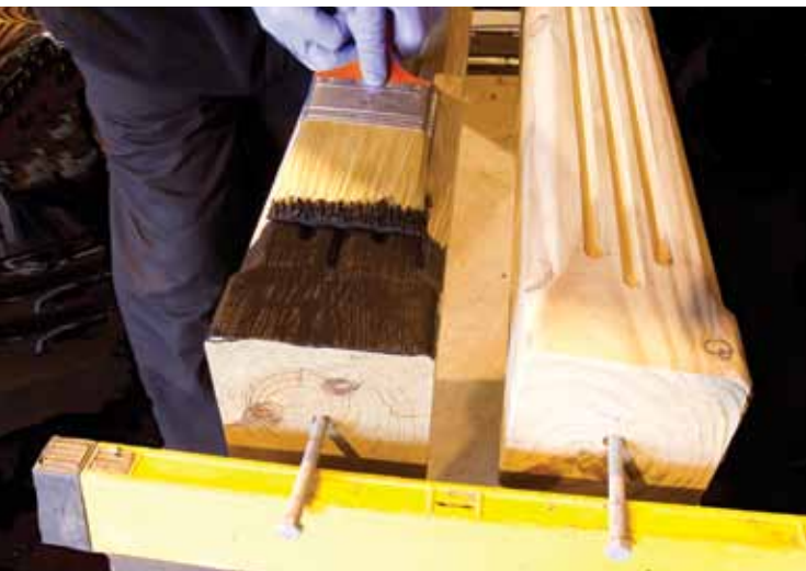
The completely milled posts are supported on shop horses by drilling holes at the top end of the posts and inserting loosely fitted, 8-in.-long lag screws. This technique permits easy post flipping during the coating process.
