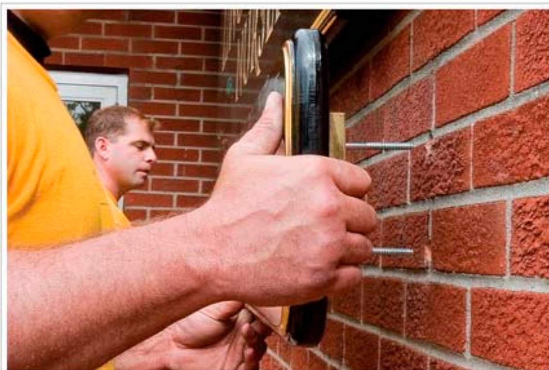
Installers insert the smaller panel with hanger bolts into drilled holes filled with 100% silicone.
