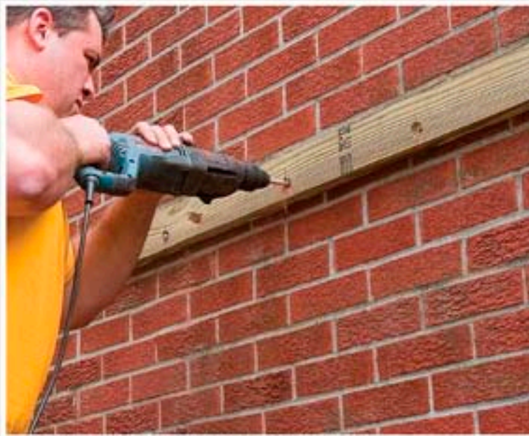
Lestingi's son, Stephen, drills holes into the brick to create space for the expansion bolts.
