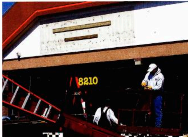
To install the sign, Francis affixed a French cleat and a treated-pine spacer for stability.
