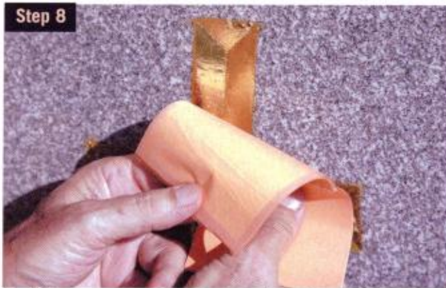
Step 8 A stiff breeze eventually precluded using a gilder's tip. Thus, Francis gingerly rolled the sheets from the goldleaf book directly onto the monument.
